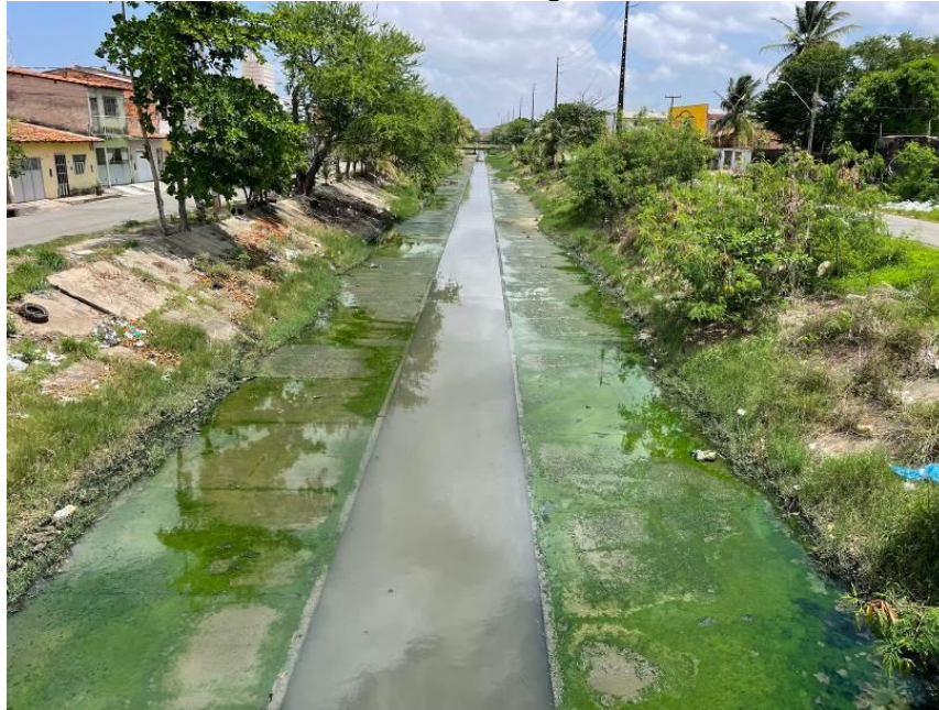
Figure 5. Drainage channel located near a Sewage Pumping Station (SPS) under construction on Avenida dos Africanos, highlighting inadequate infrastructure and visible impacts of liquid and solid waste discharge.
